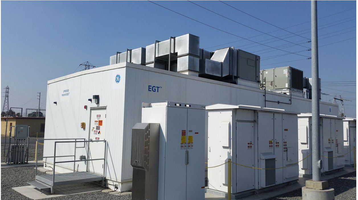
Hybrid Battery Storage System (Image by Ysc Usc)
